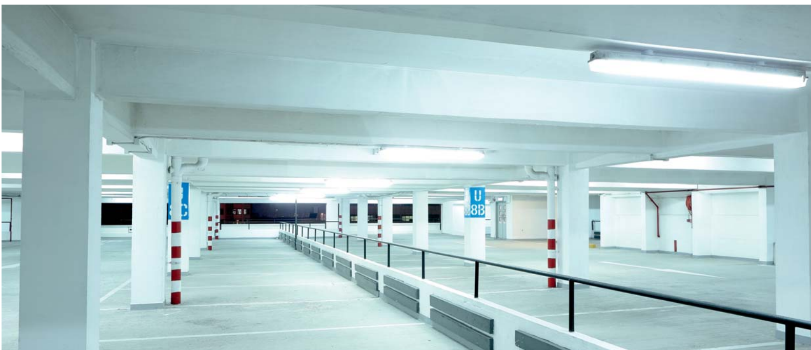
Lights for moisture-proof applications – interior application – basement garage with AL60
